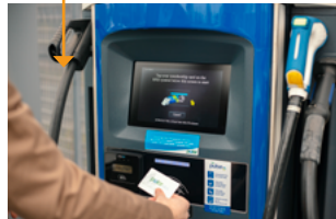
Charging point reader
